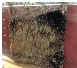
Surface coated with anticorrosive paint
